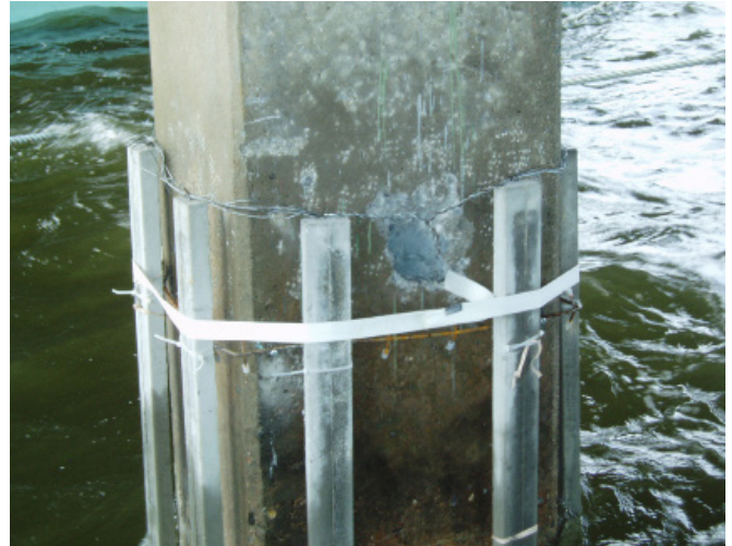
Galvanic anode system on bridge column prior to encasement in concrete jacket
